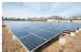
太陽光発電設備 Photovoltaic Facility
