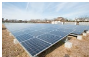
太陽光発電設備 Photovoltaic Facility
